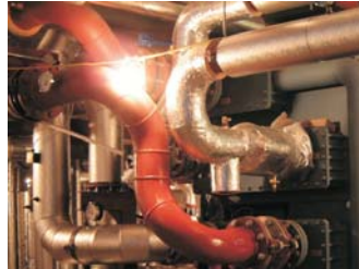
Management School Absorption Refrigeration Plant
