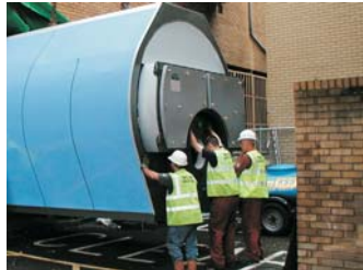
New 5 MW boiler to serve campus district heating scheme
