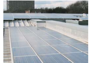
75 kW solar PV array at the Chapel development, Southampton
